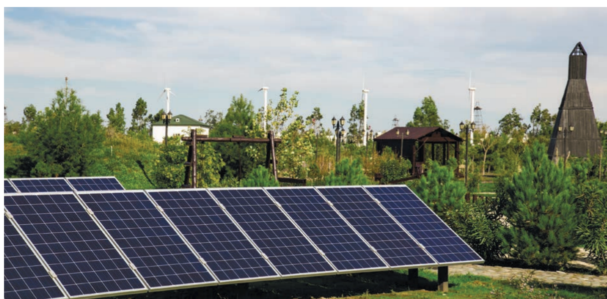
Figure XVI.1. Solar panels in Ecological Park
